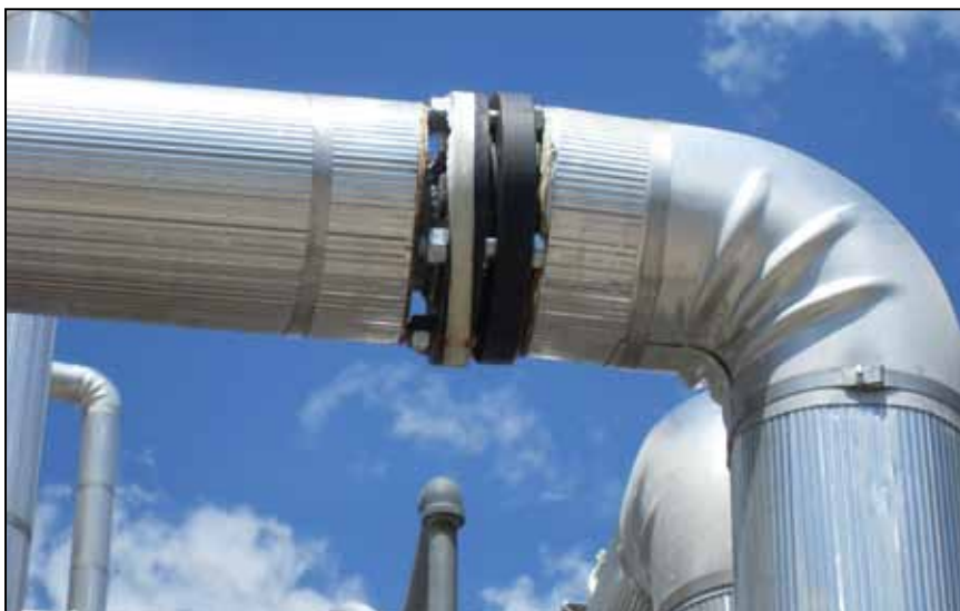
FIGURE 3. Pipe flanges are potential sources of leaks. Design considerations are important here
