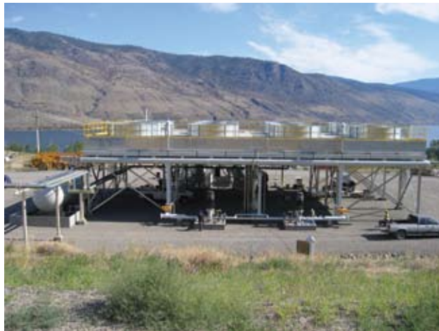
Savona ERG® facility: Organic Rankine Cycle Air Cooled Condenser
