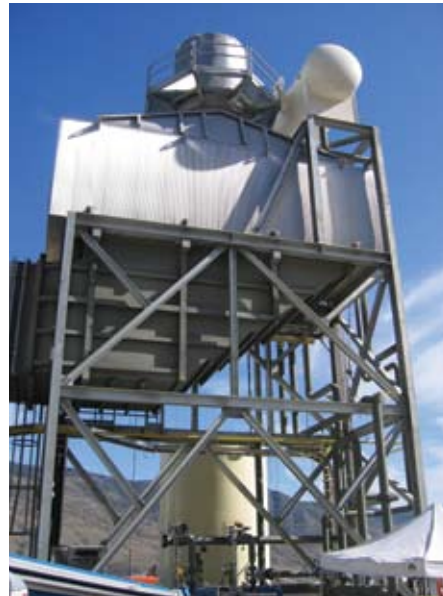
Savona ERG® Facility: Waste Heat Oil Heater
